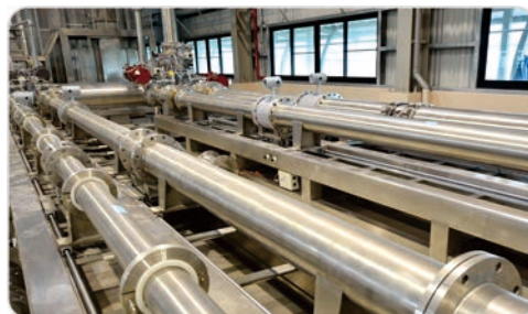
Piping system II (Maximum diameter is 300mm)
