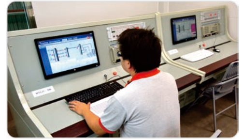
Control room & Graphical HMI
